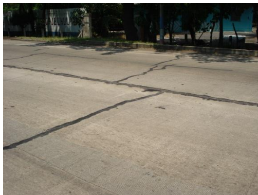
Figura 2.15 Fisura Transversal o Diagonal
